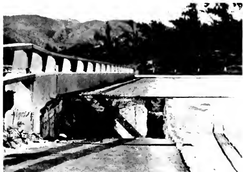
Photo 24. Differential settlement of backfill of abutment, Roxford Street undercrossing of Foothill Freeway [35].
